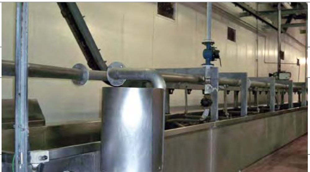
40 m s/s scalding tank with return system. Complete with pumps and overhead hanging system.
