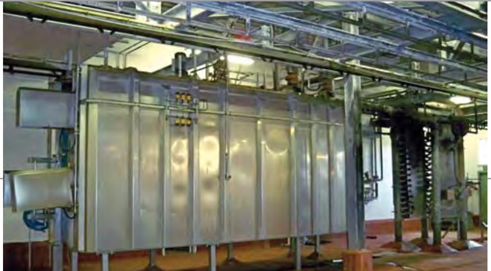
Shown on the right is the approx. 60 burner singer and final flaying and wash system.
