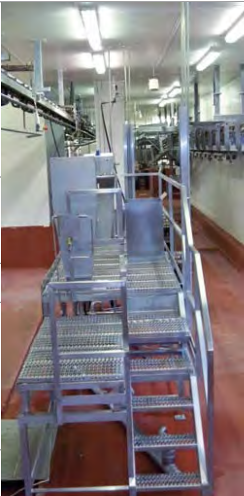
One of the many free standing work stations throughout the plant.
