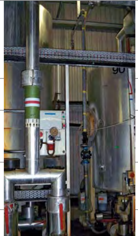
Two of the steam boilers. Three in total. Design temp 160 deg, 6 bar working pressure, tested to 9 bar. With heat exchangers for feeding the scalding tank.
