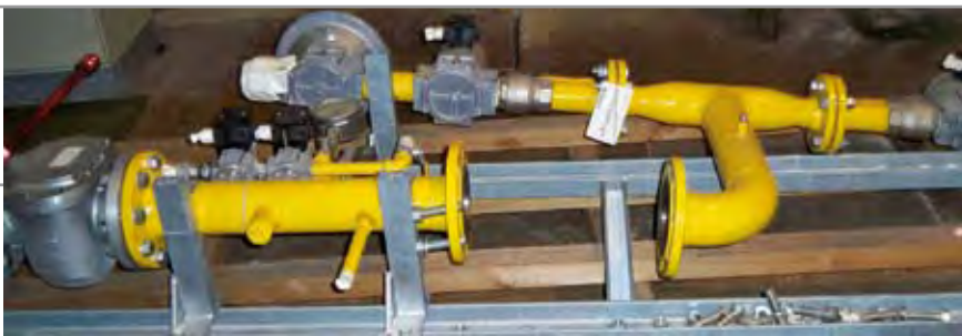
Some of the spares. New gas pipe system for singer, shown.
