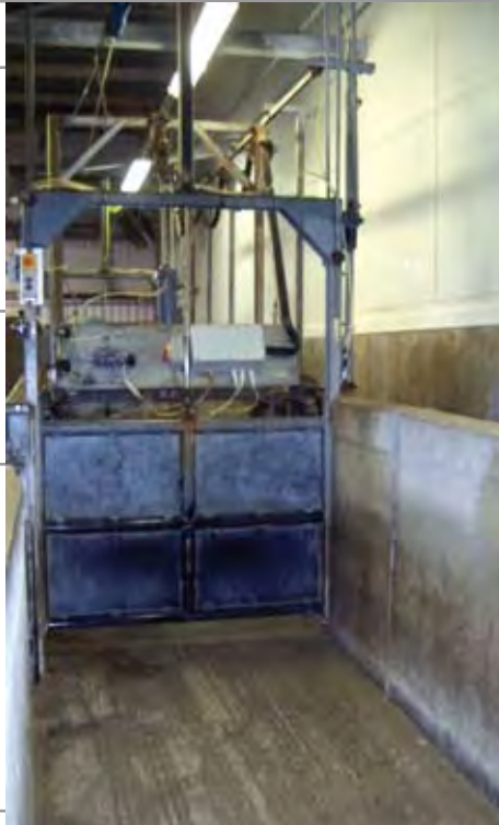
Butina auto drive system with push hoist gates. Fully automatic.
