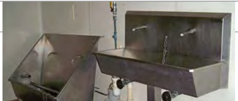
Knee operated sinks and work stations throughout the plant.
