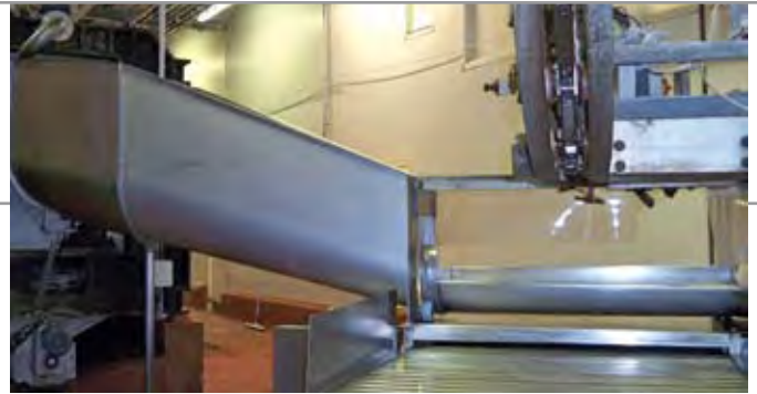
Chute feeding onto primary dressing table and shackle load system.
