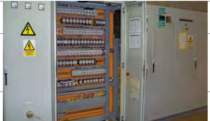
Complete control console for the whole of the line. If individual items are purchased, appropriate electrics will be separated from the panels. The whole line is variable speed.
