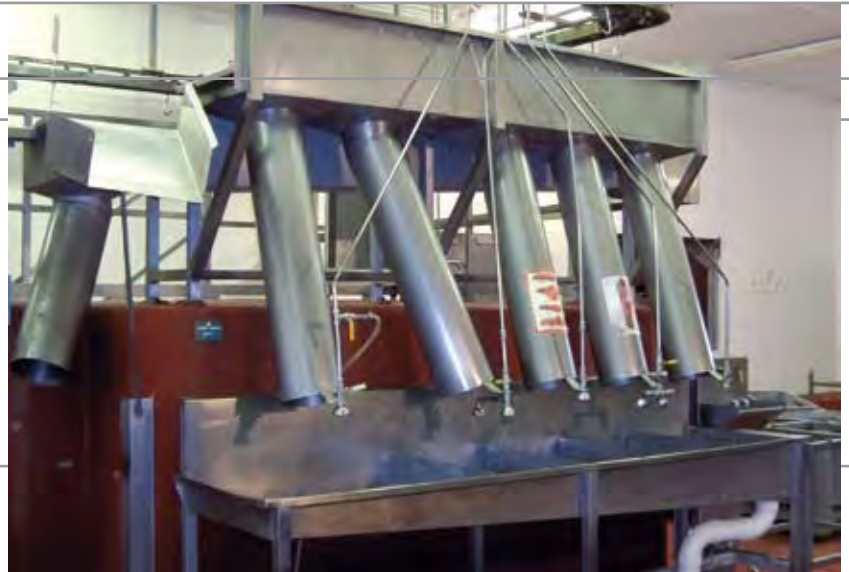
Offal sorting station chutes and work stations.
