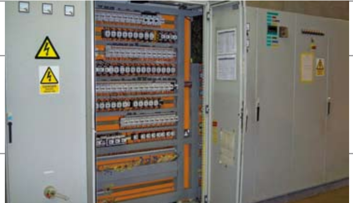
Complete control console for the whole of the line. If individual items are purchased, appropriate electrics will be separated from the panels. The whole line is variable speed.
